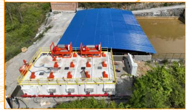
06 钻井泥浆站 Liquid Mud Plant
