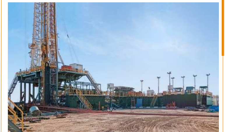
▼ 2000hp Drilling Rig Mud System
