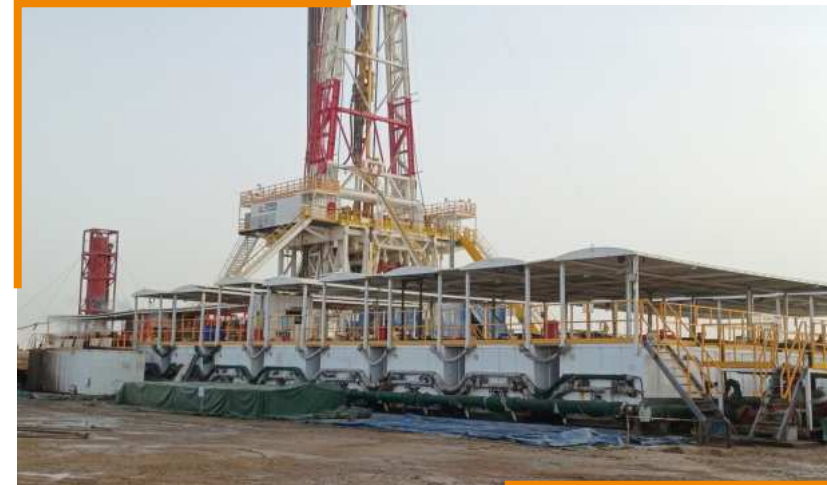
▼ 3000hp Drilling Rig Mud System
