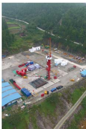
SDYJ225D operating at Fuling shale gas (skid-mounted stand-alone type)
