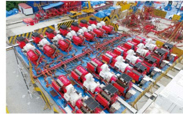
SYLQ8000Q Electric fracturing skid
