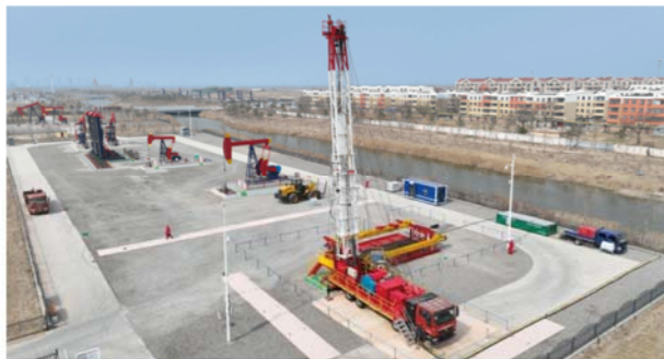
XJ350 Battery energy storage workover rig
