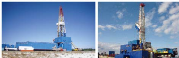
ZJ50DT cold-weather train-rail type drilling rig is working for EuroAsia in RUSSIA
