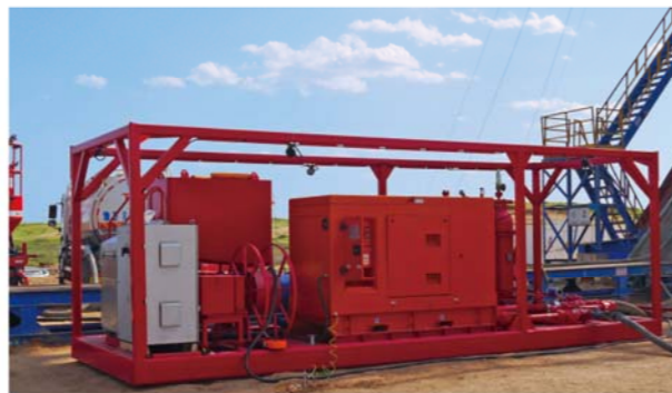
SPH14-7 Foam slurry mixing skid work in Wushenqi
