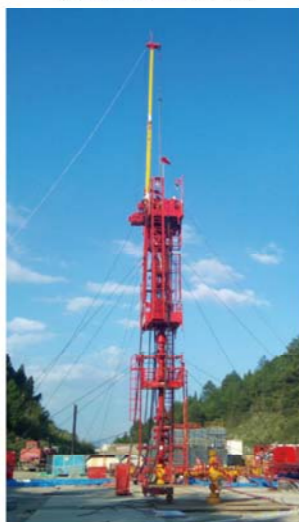
SDYJ160D operating at Fuling shale gas (skid-mounted stand-alone type)
