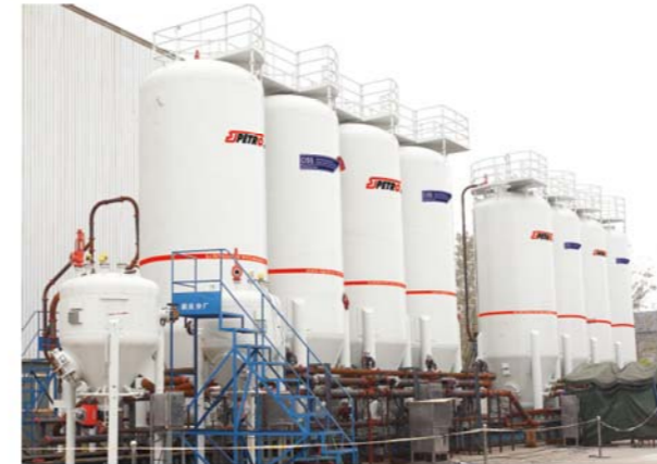
Cement tank and bulk system
