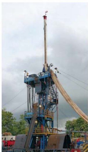
SDYJ160D operating in Thailand (skid-mounted stand-alone type)
